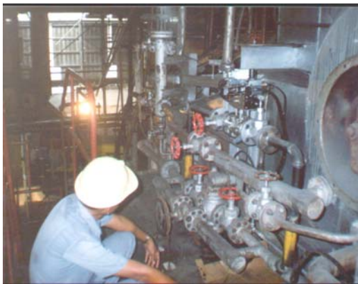
Monitoring the control valve action
